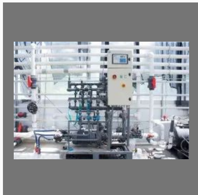
Open Field Irrigation Controller
