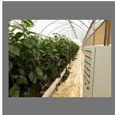
Roof Top Controller
