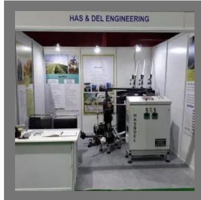
Agriculture Fully Automatic Fertigation System
