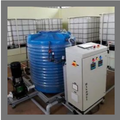
Automatic Fertigation System with Dosing Pumps
