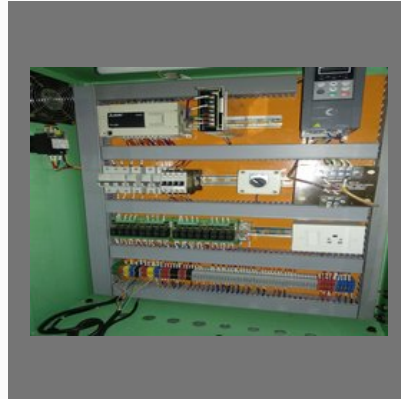
PLC Based Electrical Control Panel Box
