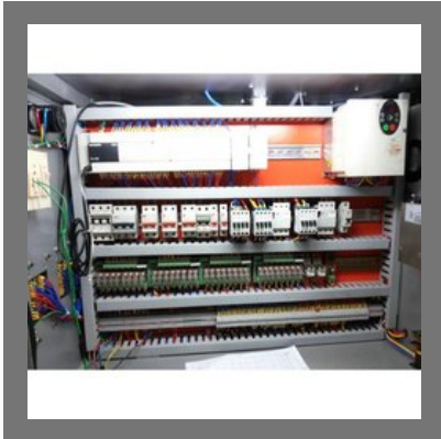
PLC Based Control Panel Box
