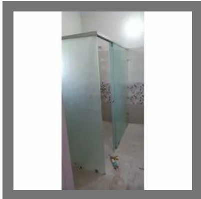
Bathroom Glass Shower Enclosure
