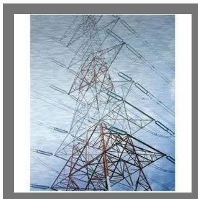
Transmission Line Towers
