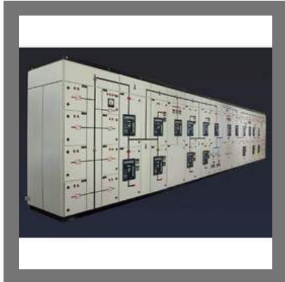
Sub Station AMC
