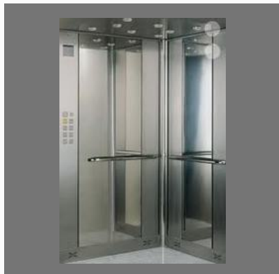
Operation & AMC of Lifts
