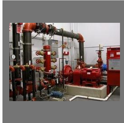
Service and Installation of Fire Fighting Equipments
