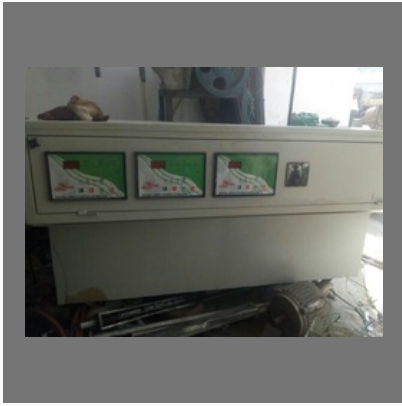
Control Panel 1080 V
