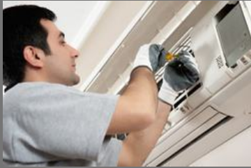
Home Electrical Installation Service
