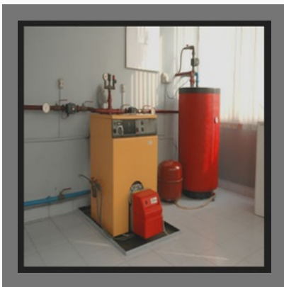
Burner And Boiler
