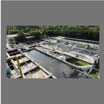
Effluent Treatment Plants
