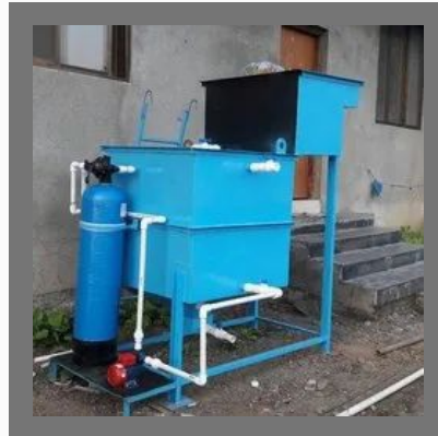
Sewage Treatment Plant Services
