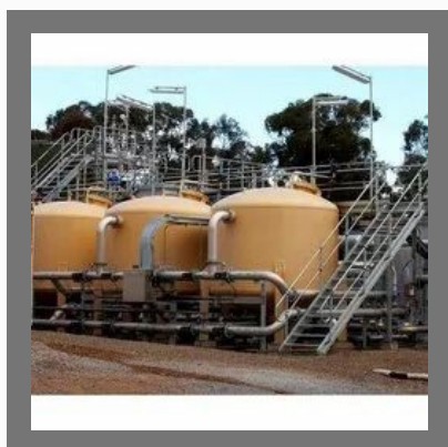
Commercial Sewage Treatment Plant
