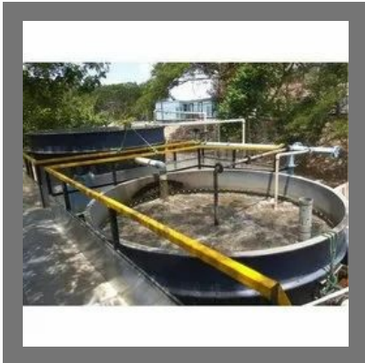
Domestic Sewage Treatment Plant Service
