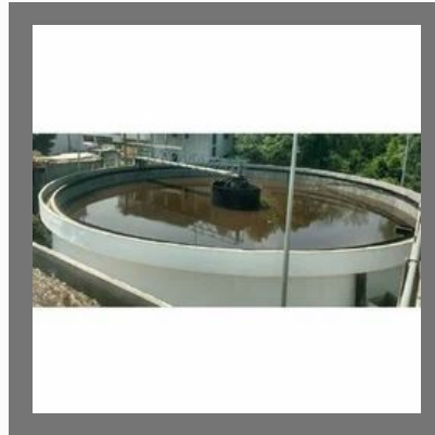
ETP and STP Plant
