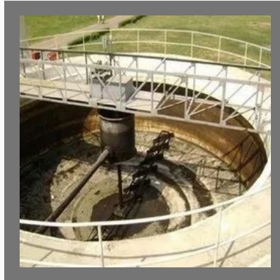
Effluent Treatment Plant And Maintenance Services
