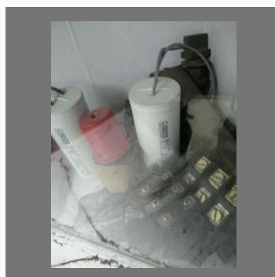
Industry Electrical Capacitor
