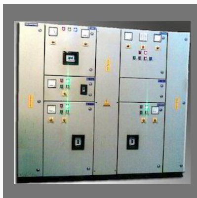
Motor Control Center
