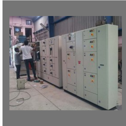
Power Distribution Panel
