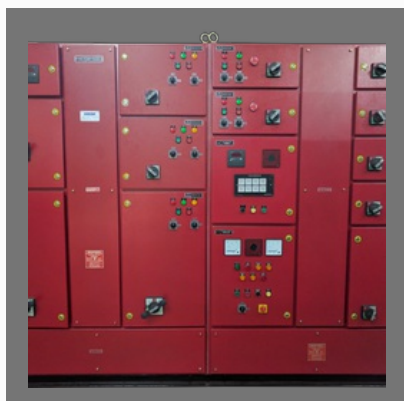
FIRE FIGHTING PANEL
