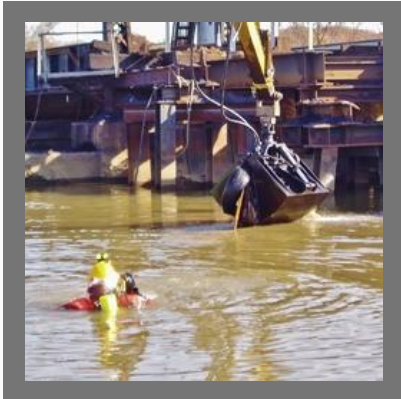
Underwater Feed Pump Inspection Service
