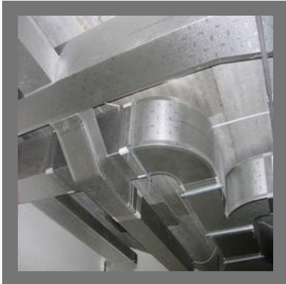
Duct Fitting Services
