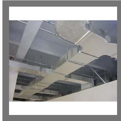
Air Conditioning Duct
