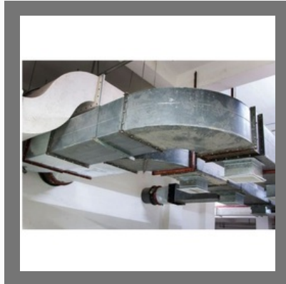
Air Conditioning Ducting Service
