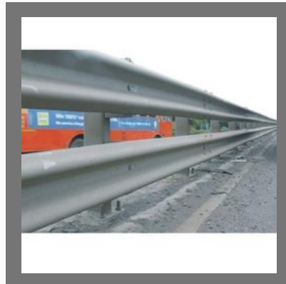
Single Sided Double Metal Beam Crash Barrier
