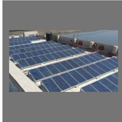
Industrial Solar Power Plant
