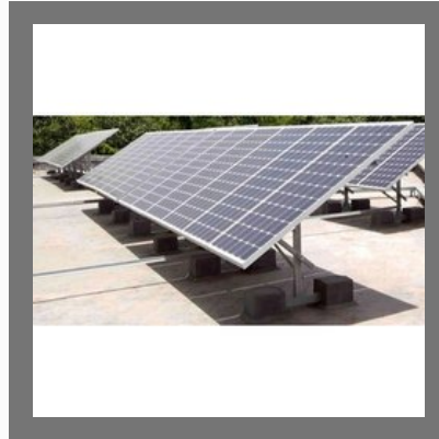
Off Grid Solar Power Plant
