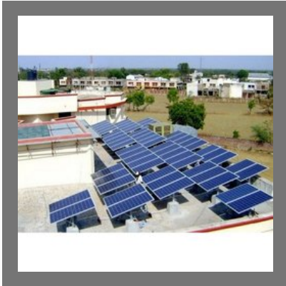
Roof Top Solar Power Plant
