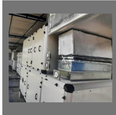
Air Handling Unit
