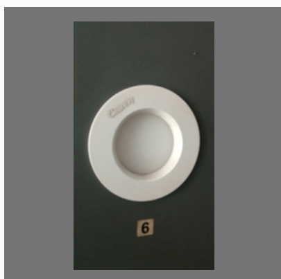
LED Ceiling Lights
