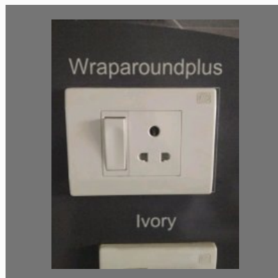
Electrical Switch Board
