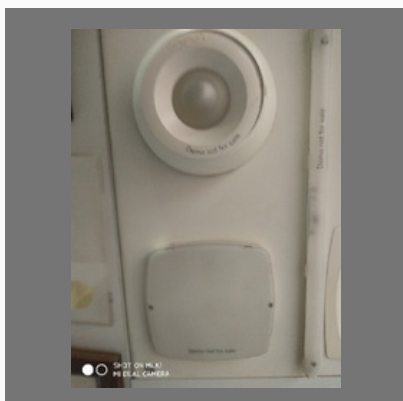
LED Ceiling Lights
