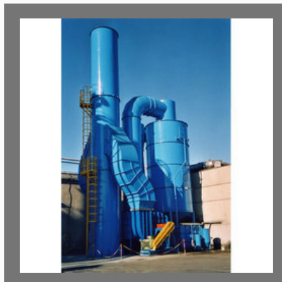
Wet Scrubber System
