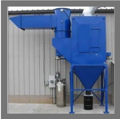
Dust Collection System
