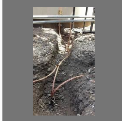
Lightning Protection System
