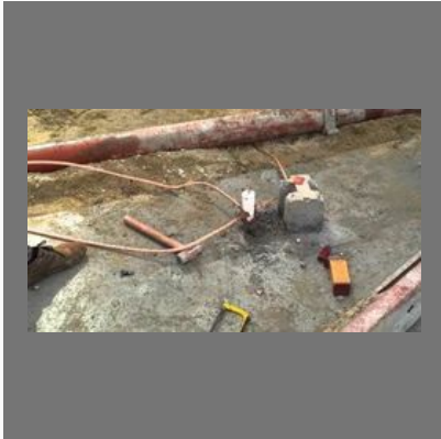
Chemical Earthing System
