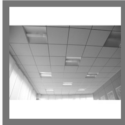
Grid False Ceiling
