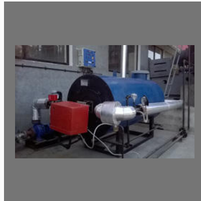
Oil Fired Hot Water Generator-Operating Temp 90c
