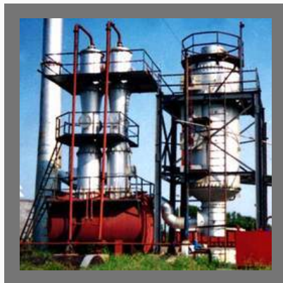
Vertical Liquid Incinerator-30 000 Liters Per Day With Twin Scrubber
