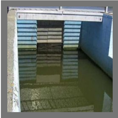
De Chlorination Chemicals
