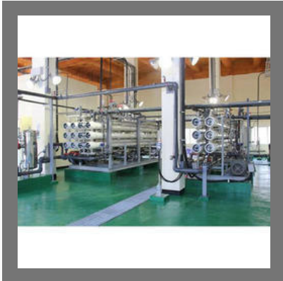
Industrial RO Plant
