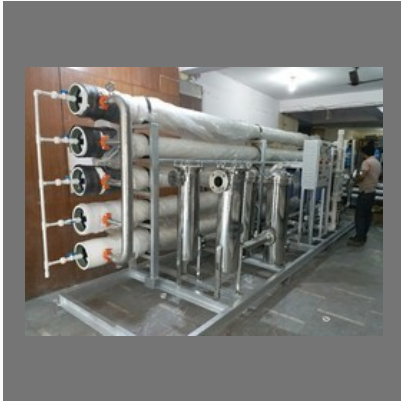
R.O. Plant 25 m 3 / Hr
