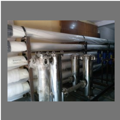
Reverse Osmosis Plant
