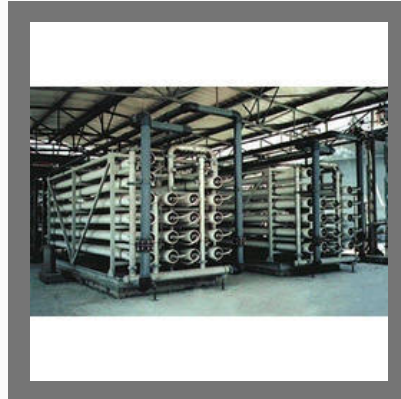
Reverse Osmosis Plant
