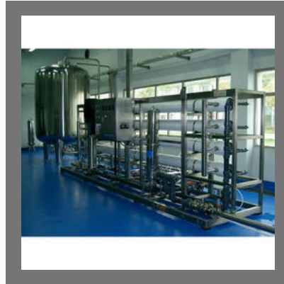
RO Water Plant 20M 3 /Hr
