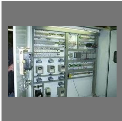
Allen Bradley PLC
