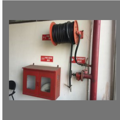
Fire Fighting System
