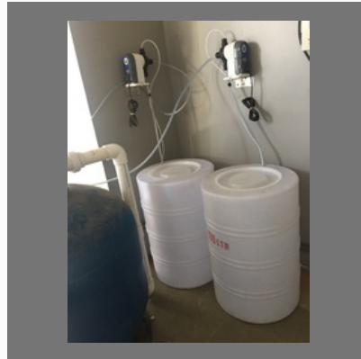
Chemical Dosing Pump
