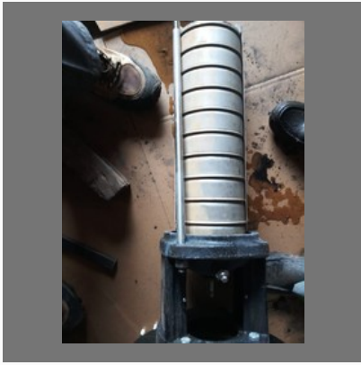
High Pressure Pumps
