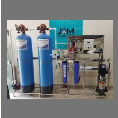
Reverse Osmosis Plant
