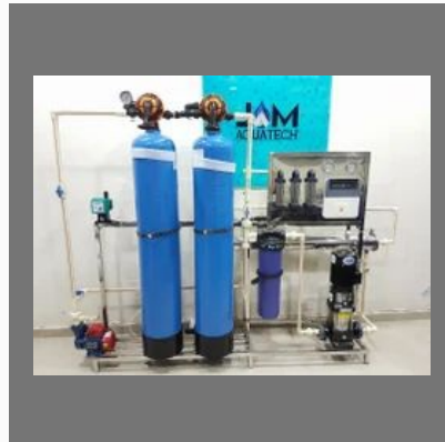
Industrial Reverse Osmosis Plant
