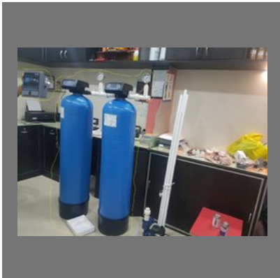
Automatic Softener and Sand Filter
