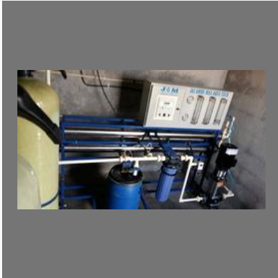
Drinking Water Treatment Plant
