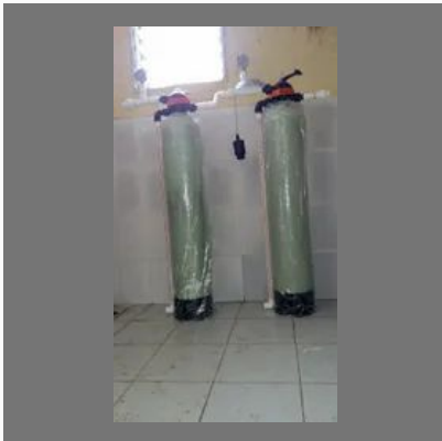
Bathroom Water Softener
