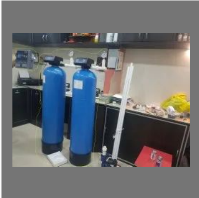
Water Softner Plant
