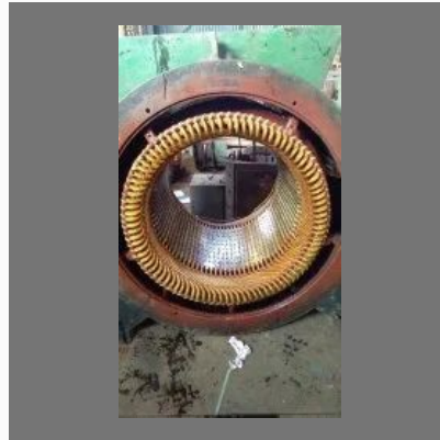
AC Motors Rewinding HT 6.6 KV
