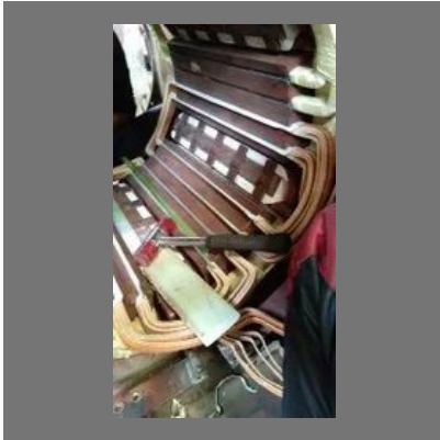
DC Motor Rewinding Services 145 KW C/F Machine
