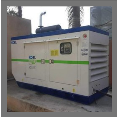
25 kVA Koel Green Diesel Generator
