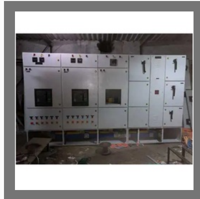
Digital Control Panel
