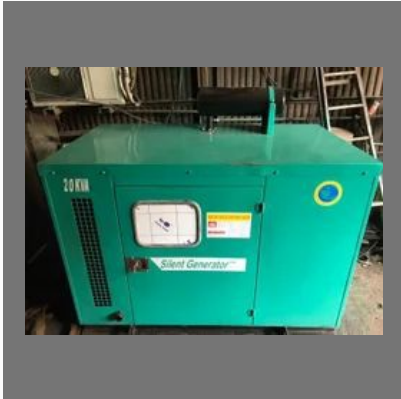
20 KVA Silent Diesel Generator
