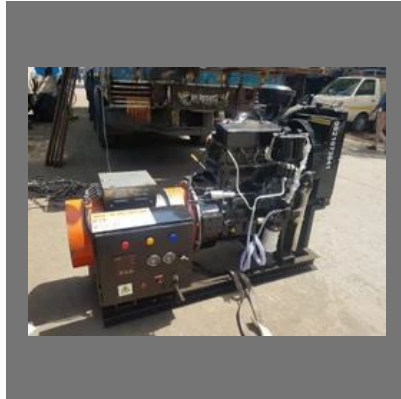
40 Kva Open Generator
