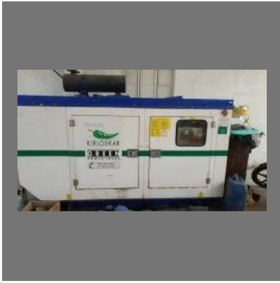
Kirloskar Diesel Generator
