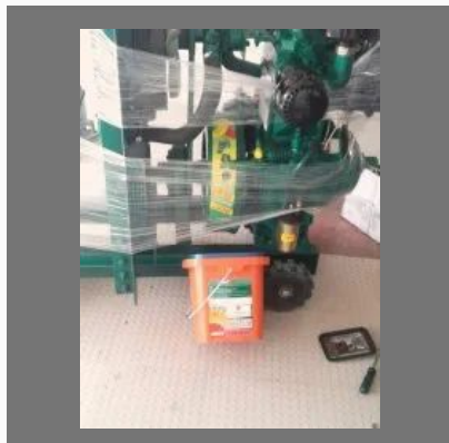
Diesel Engine Generator
