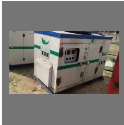
Kirloskar Diesel Generator
