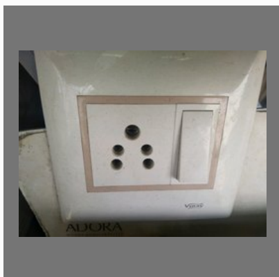
Electrical Switch Board
