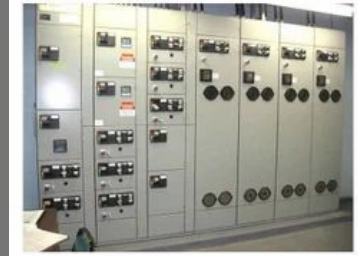
Electrical Control Panel Service
