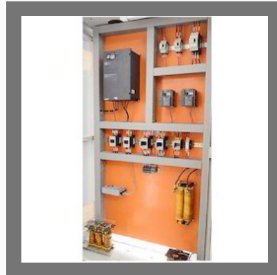
VFD Panel Electric Enclosures
