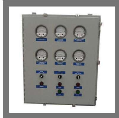
Pneumatic Control Panel Enclosure
