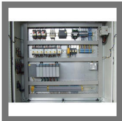
PLC Panel Electric Enclosures
