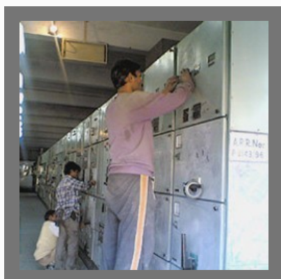
Control Panel Maintenance Services
