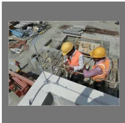
Lightning Protection System
