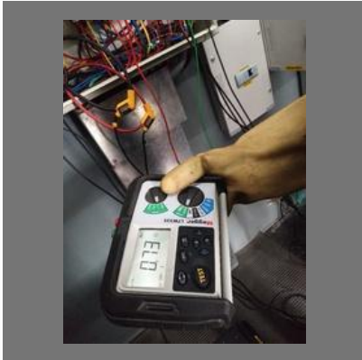
ELECTRICAL SAFETY AUDIT
