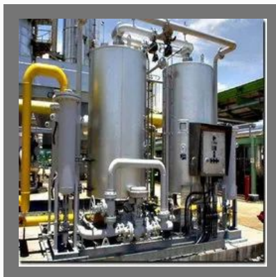
Gas Dryer Package
