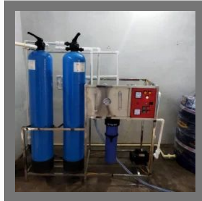
250 Lph Industrial Ro Plant
