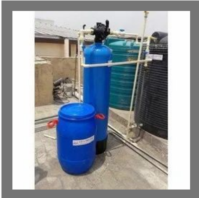
Water Softener Plant
