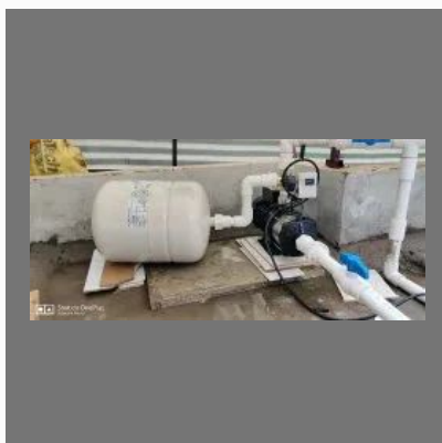
Water Pressure Pump
