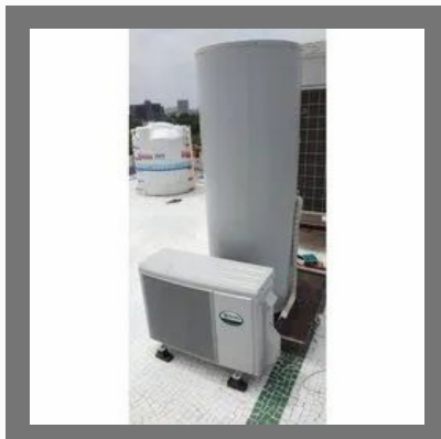
Heat Pump Water Heater
