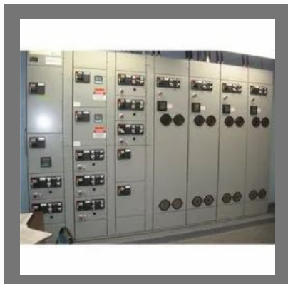
Three Phase Electrical Panel
