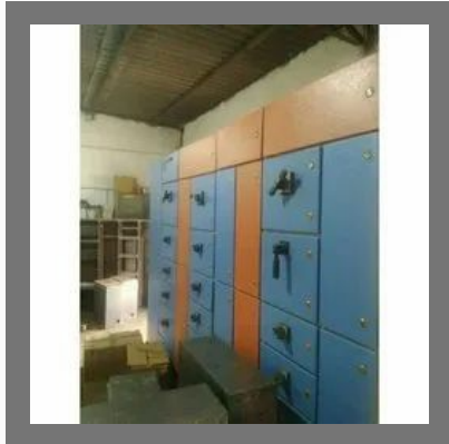
Three Phase Distribution Panels
