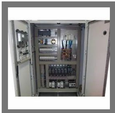
PLC Automation Control Panel
