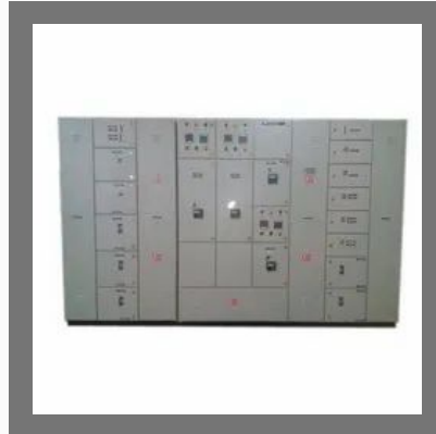
Power Distribution Panels
