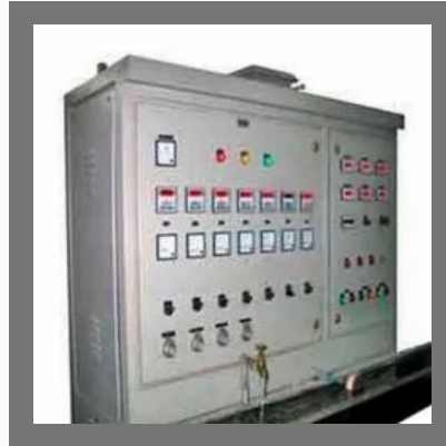
Control Panel Board
