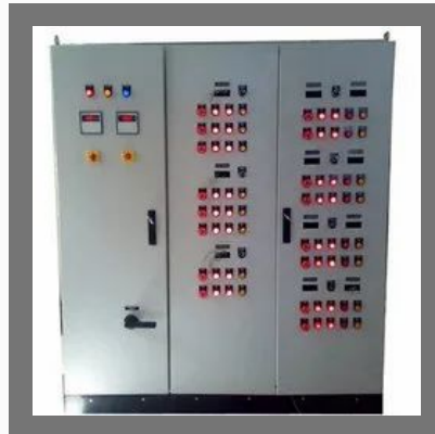
Cold Room Control Panel
