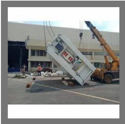
Heavy Job, Machinery, Equipment Material Handling , Loading ,Erection Of Heavy Equipment Service
