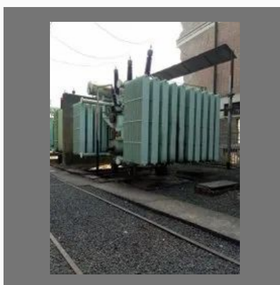
Transformer Dragging Service
