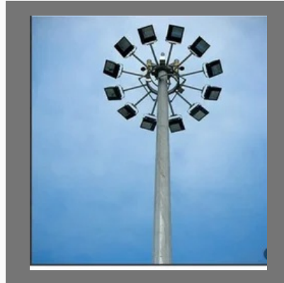
LED High Mast Lighting Pole
