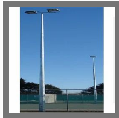
Street Light Pole
