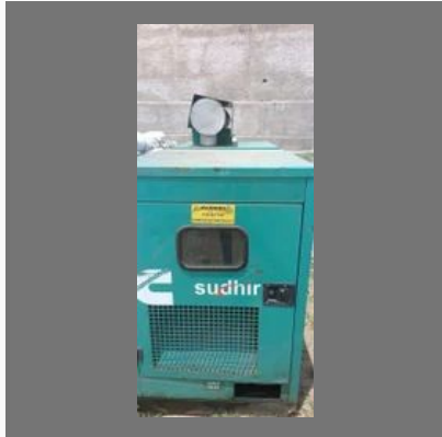
Cummins Power Diesel Generator
