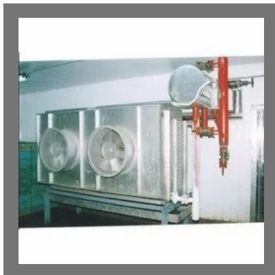
Cold Storage Installation & Maintenance Services
