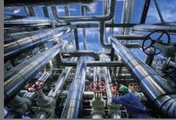
Oil & Gas Pipelines Service
