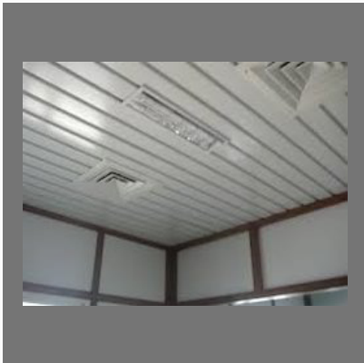
PVC False Ceiling
