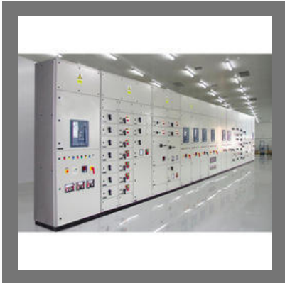
DG Synchronization Control Panel
