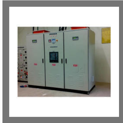
Active Harmonic Filters panel
