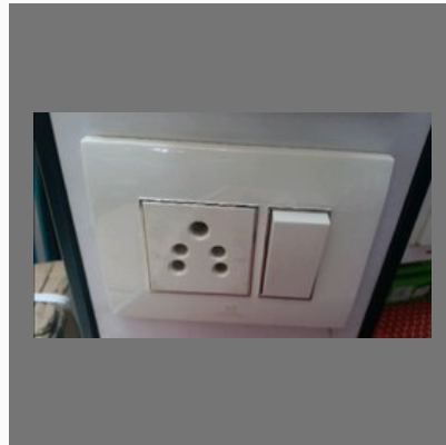
Single Modular Switch Board
