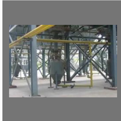
Pneumatic Conveying System
