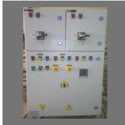
AC Drive Control Panel
