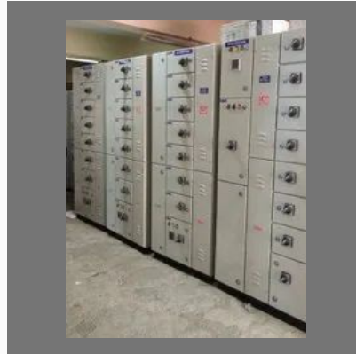
Industrial Electrical Control Panel
