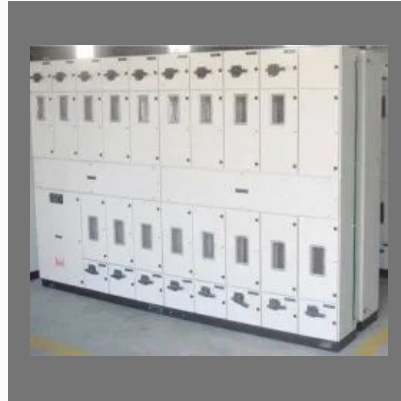
Large Electricity Board Metering Panel
