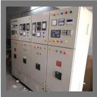
AMF Electric Control Panel Board
