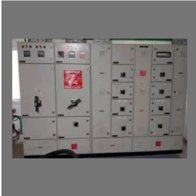
Three Phase Main Distribution Panel
